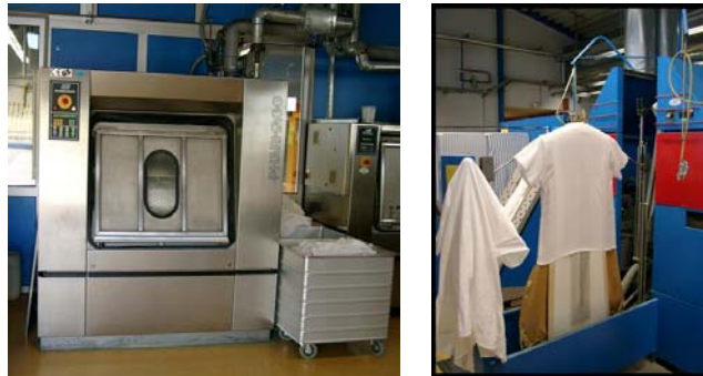
Fig 6: Laundry: Washing machine and finishing equipment.
