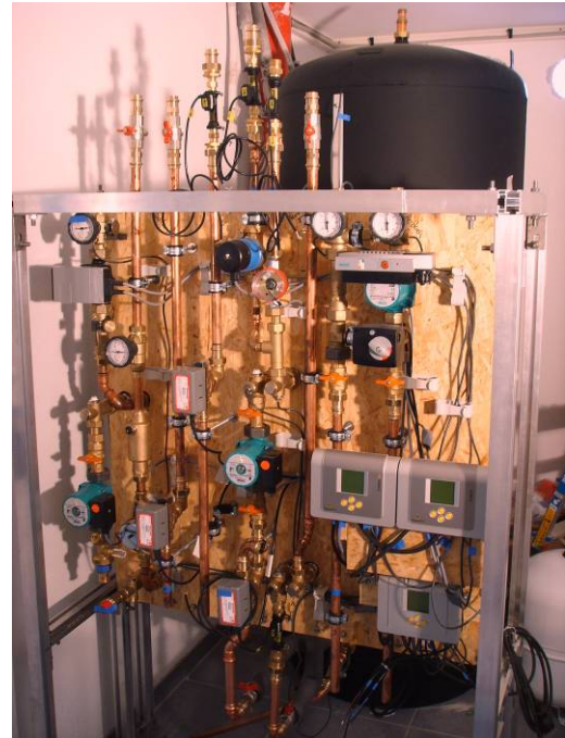
Figure 3. The single-family house with 16.8 m 2 of façade-integrated collectors (left) and the prototype of the charge and discharge unit in the basement (right) during installation.
